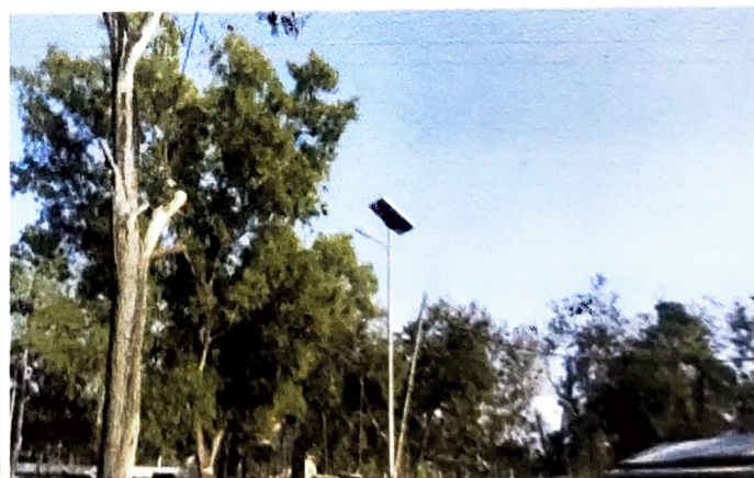
Solar Street light
