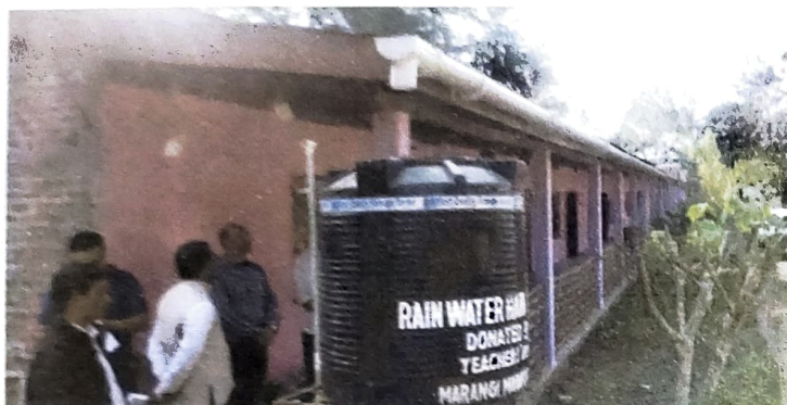
Rain Water harvesting tank
