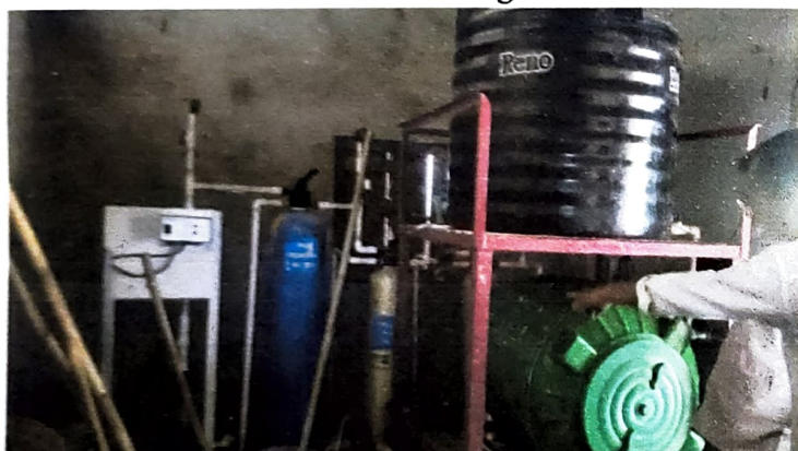
Water purifying RO unit
