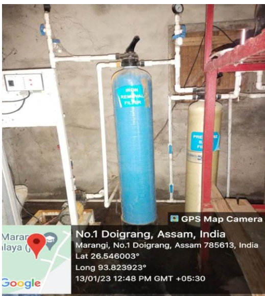
Photo-1. Water purifying plant (RO)
