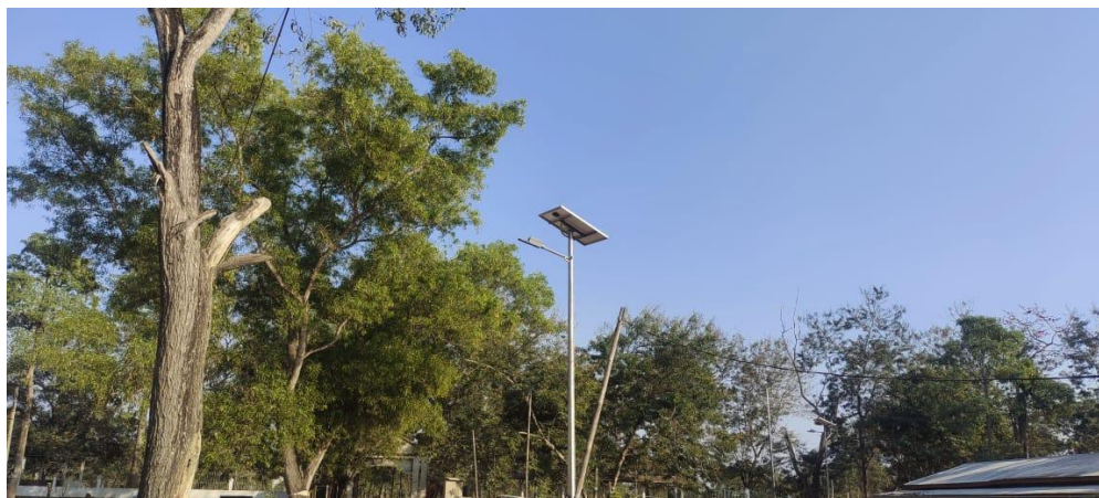
Photo-25. Solar street light in the college campus
