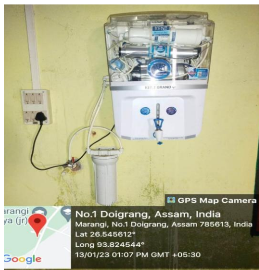
Photo-3. RO Water purifier
