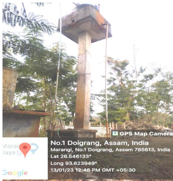
Photo-2. Overhead Water Tank for distribution
